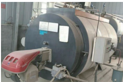
■ Air supply fan for boiler
